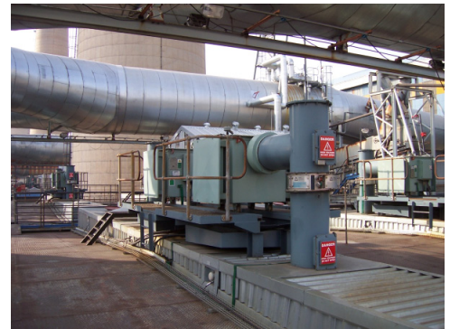
TR set with earthing device
