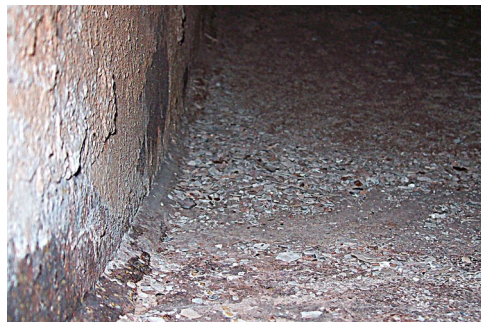
Fig 2 - Scale build-up on furnace to tube plate
