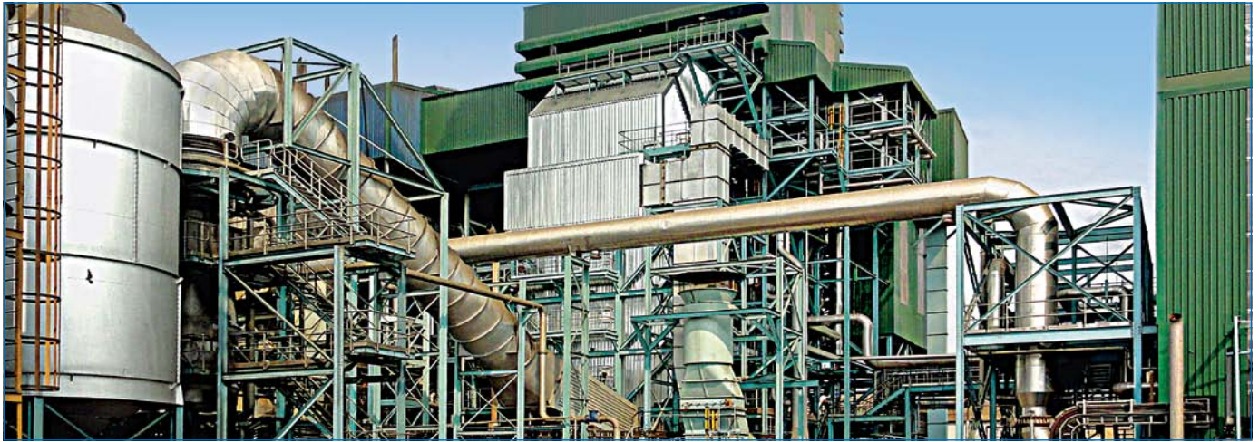
Typical sugar industry boiler
