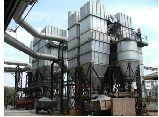
Foundry: Sand reclamation, breaker and shaker drum dedusting
