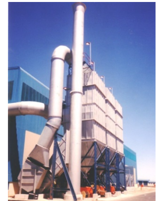
Furnace: Gas cleaning
