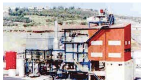
Figure 2: General view of the boiler and associated equipment.
