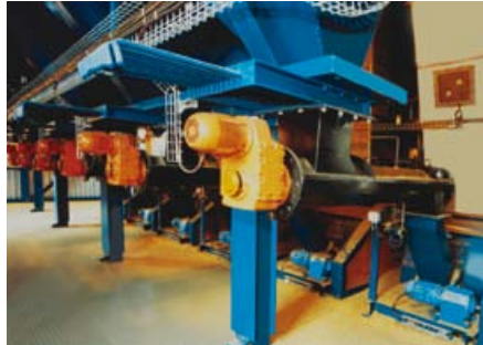
Coal & Bagasse Feeders.
