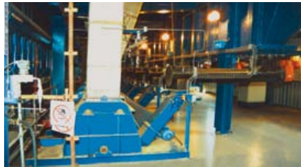
Bagasse & Coal Feeding System.
