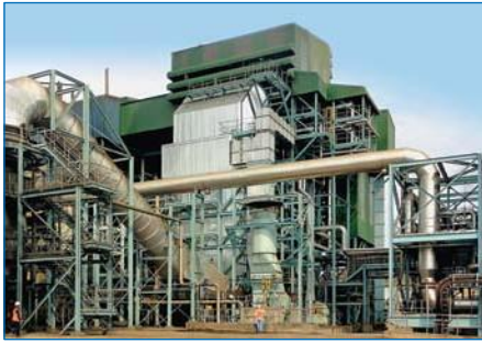
Typical sugar industry boiler
